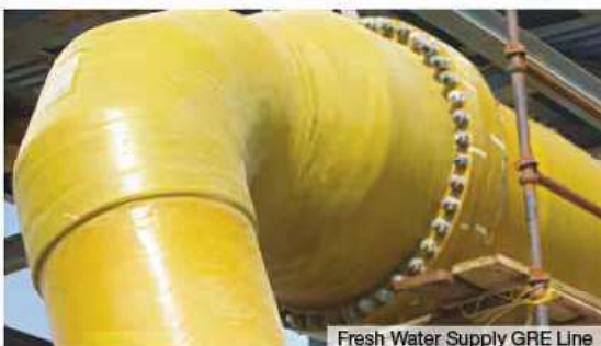
Fresh Water Supply GRE Line
