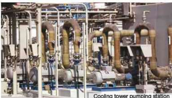
Cooling tower pumping station
